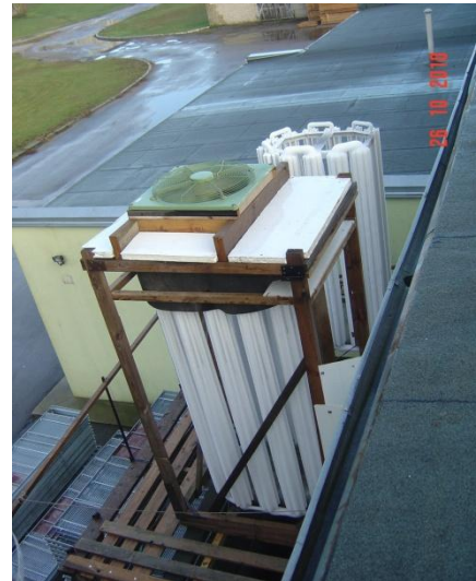
Fig.2. Ventilator above the heat pump evaporator
